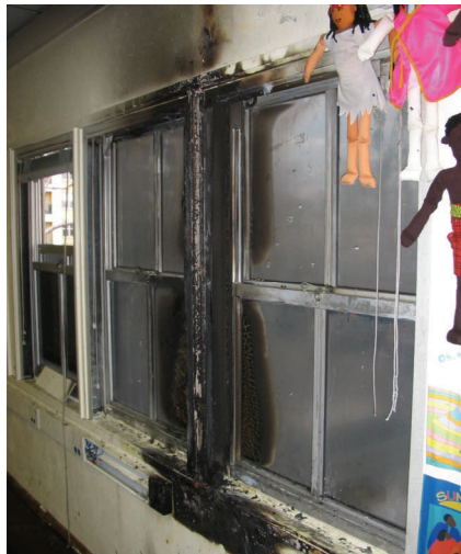
Aftermath of a recent electrical fire at LaSalle Elementary
